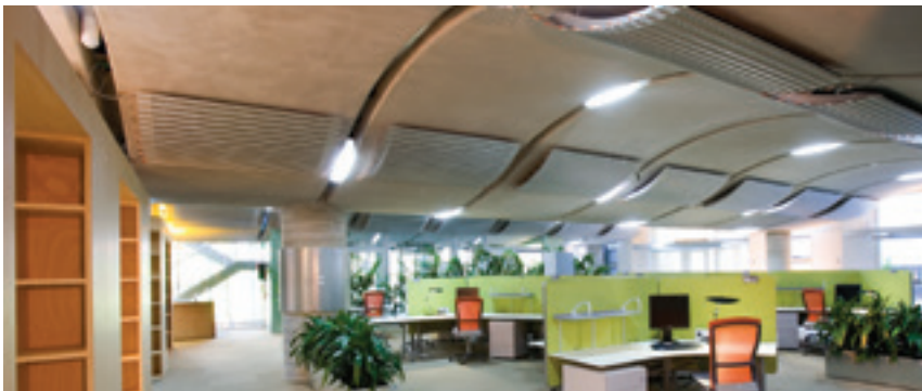
CH2 | MELBOURNE The 'displacement ventilation system' supplies fresh air to the floor at low velocity while older air is exhausted through ceiling vents on the roof.
