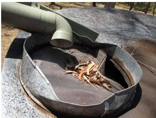
Improperly sealed rainwater tanks can become breeding sites for mosquitoes
